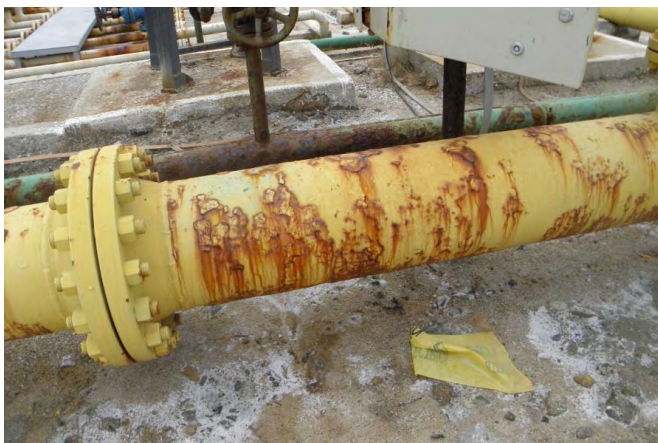
Fig. 1 - Paint breakdown and external corrosion
