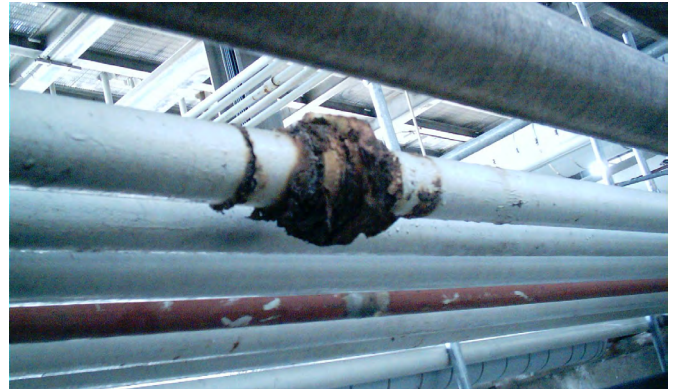
Fig. 3 - Paint breakdown and external corrosion
