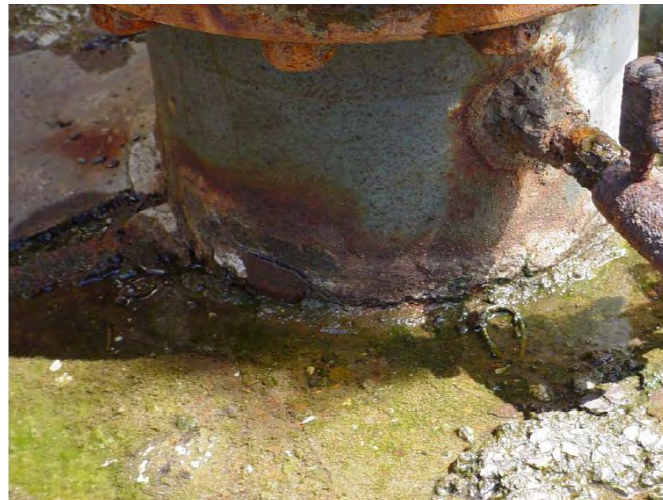
Fig. 5 - Corrosion Under Insulation
