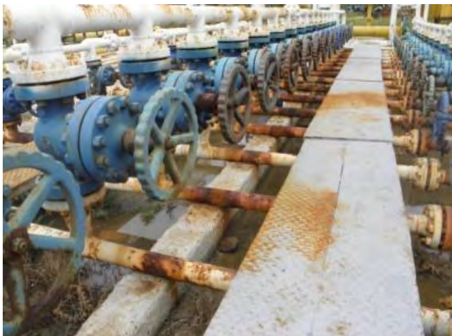
Fig. 2 - Corrosion at pipe supports
